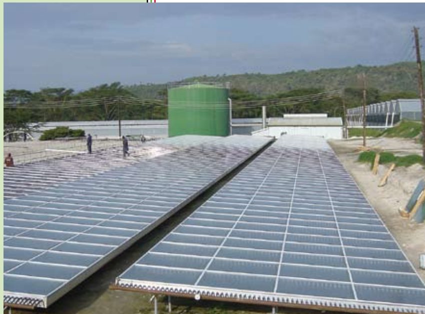
Solar panels cover a surface of 3200 m 2 , heating water up to fifty degrees Celsius in the daytime.
