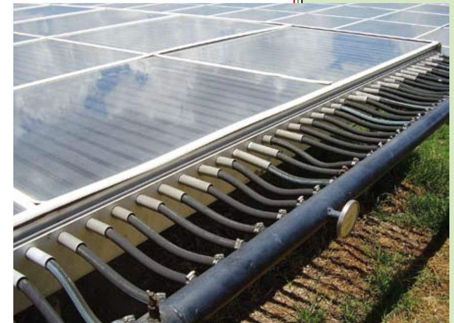
Water is pumped through blackened tubes.
