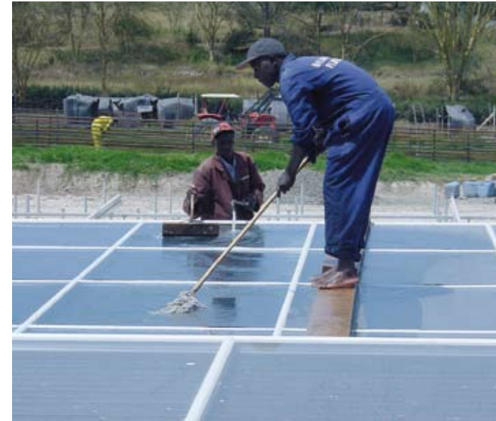
To obtain maximum transmission efficiency, cleaning the panels is essential.
